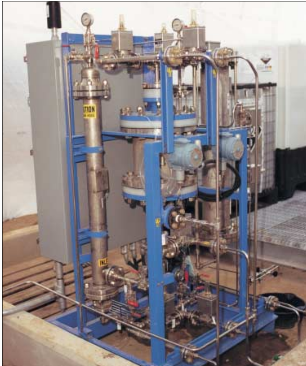
Duke Energy Field Services installed this ion-exchange reclamation unit to remove HSAS and bicine the amine.
