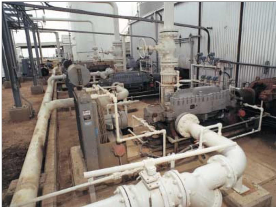
High-pressure amine circulation pumps saw the first problems at the Wilcox gas plant.
